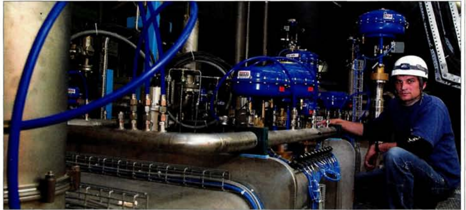
Adrien Forgeas, of the Commissariat à l'Energie Atomique (CEA), Grenoble, one of the team responsible for supervising the installation and commissioning the cryogenic unit at Point 8.
